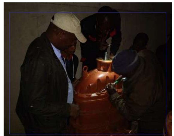
The Technical team burning the midnight oil to ensure supply resumes after cleaning the clear water tank
