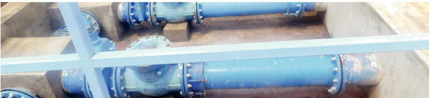
Piping at King'ong'o Pumping Station
