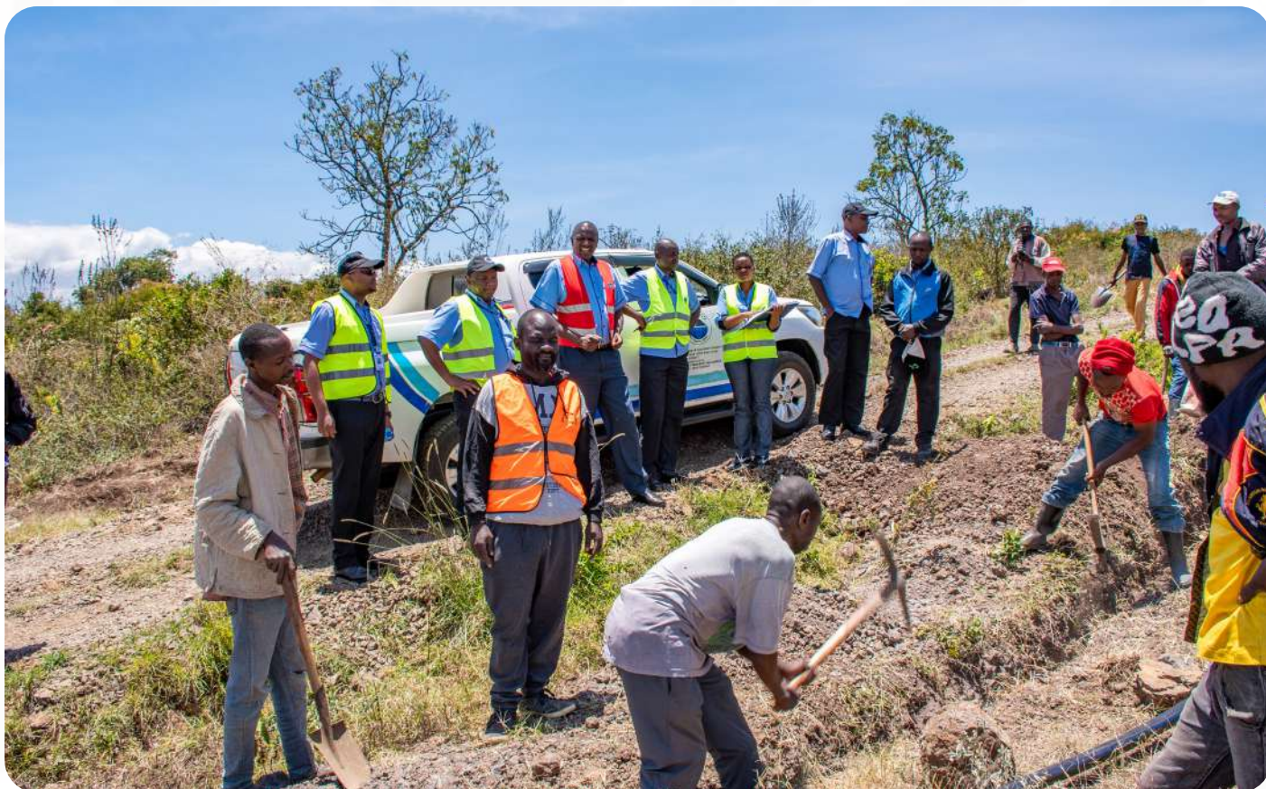
NYEWASCO Management team at an ongoing water extension project, assessing progress and quality to ensure timely and sustainable service delivery.
